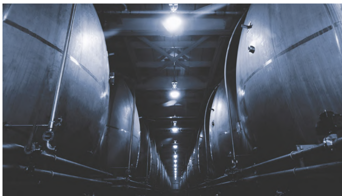
Fill level measurement in tanks
